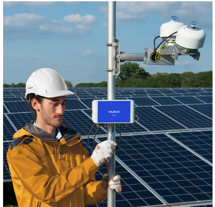
Figure 8 Two SR300-D1 pyranometers that are connected to the SPD01 Surge Protection Device. With the optional SPD01, you can upgrade surge immunity to level 4.
