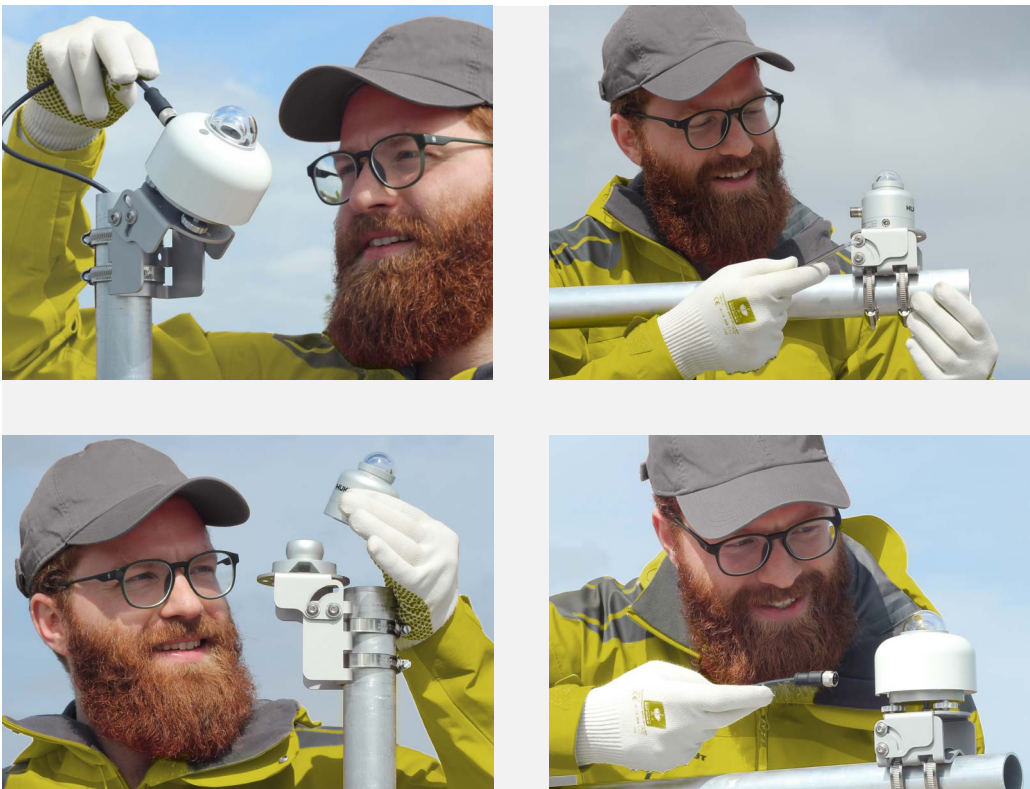
Figure 0.4 Hukx pyranometers with PMF01 pyranometer mounting fixtures on a horizontal crossarm and on a vertical mast, being installed both in Plane of Array (tilted) and horizontally. The versatile PMF01 allows for mounting on a surface, using bolts, as well.
