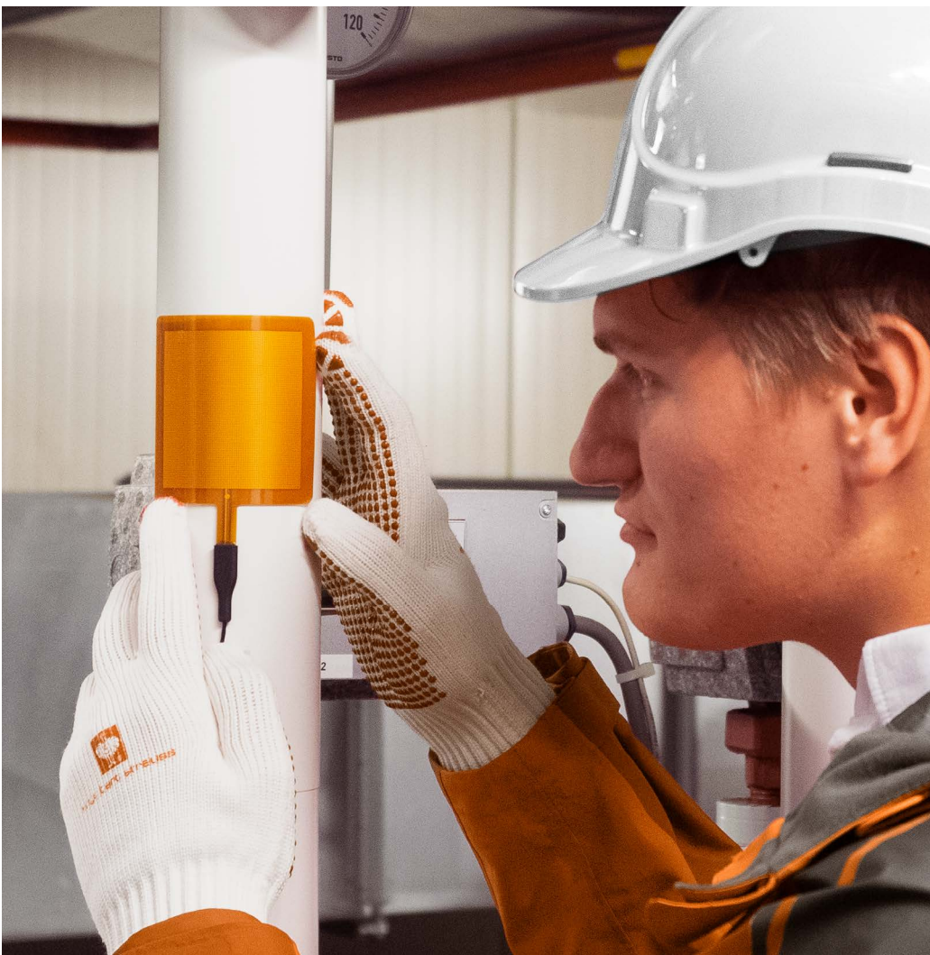
Figure 2 FHF05-85X85 being installed to measure heat flux on a pipe.
