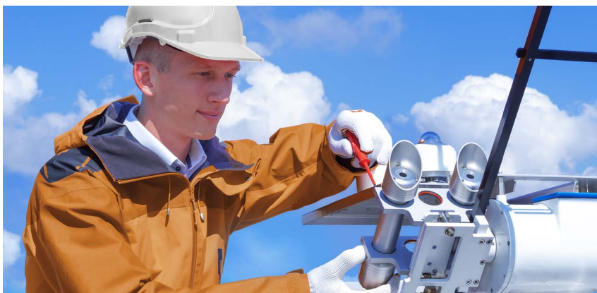
Figure 0.2 Application of DR20-A1 and DR15-A1 pyr heliometers, here with SR15-A1 pyranometers, in a typical solar radiation monitoring station.
